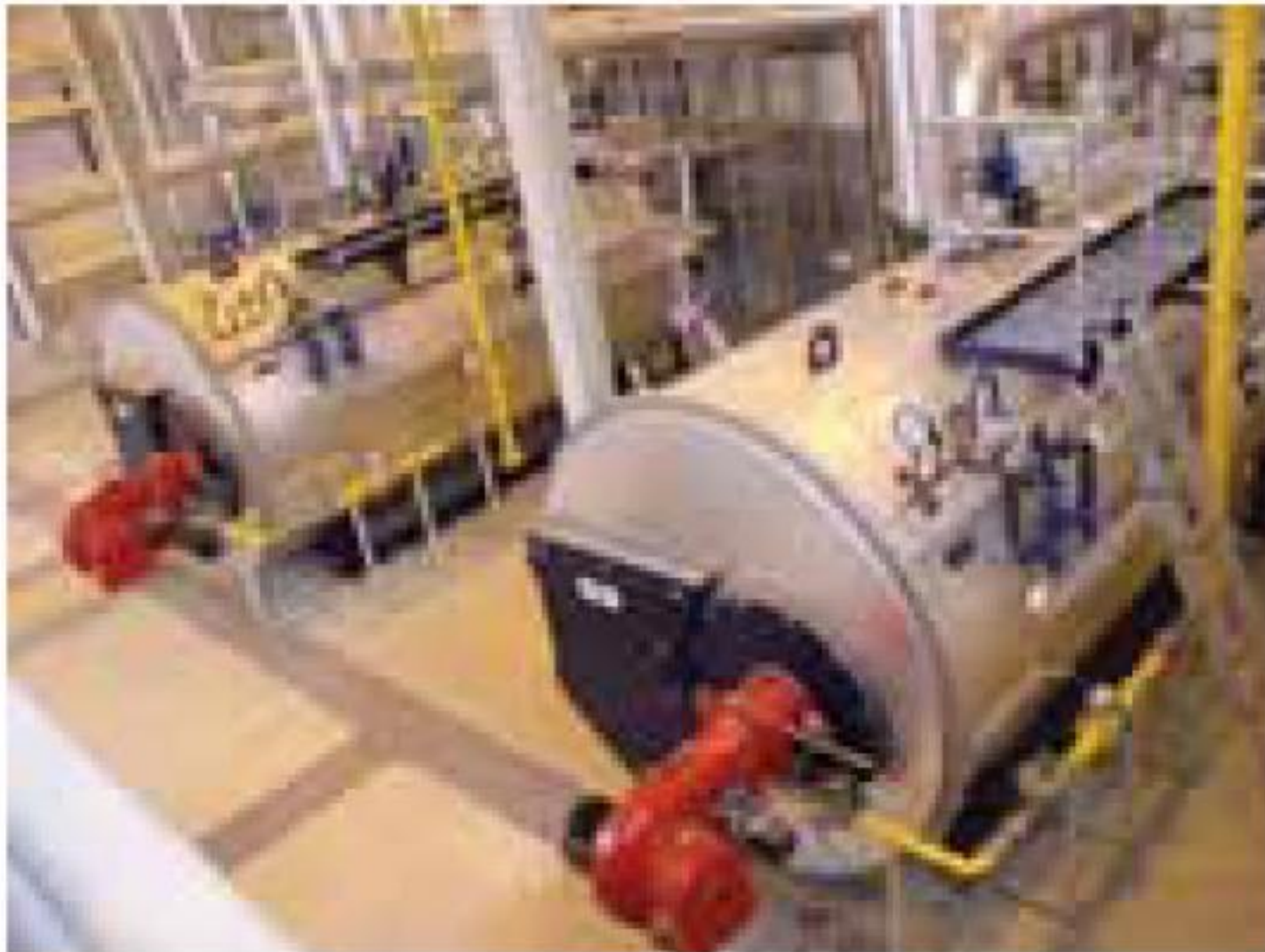
Boilers in a plant. A good boiler should efficiently take the heat from the fuel and minimise loss of heat from inside to outside.
