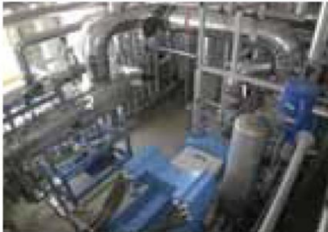
Pipework inside a factory.
