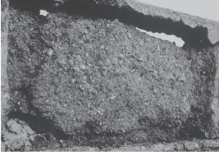
Figure 5.21 An example of a degraded 'mundic' block.
